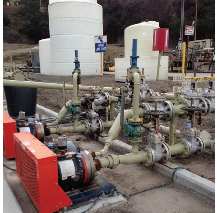
Several operational features of Hydra-Cell pumps are showcased when processing volatile crude oil.
