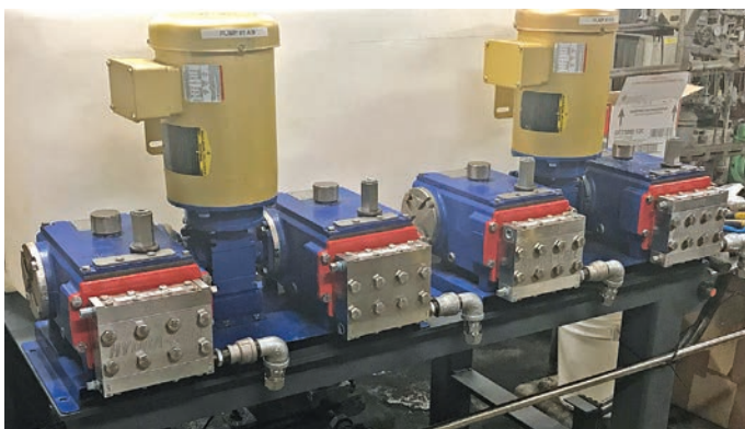
Chemical boiler feed at a power plant. Four MT8 pumps running off two gearboxes and two motors shows its duplexing capability.
