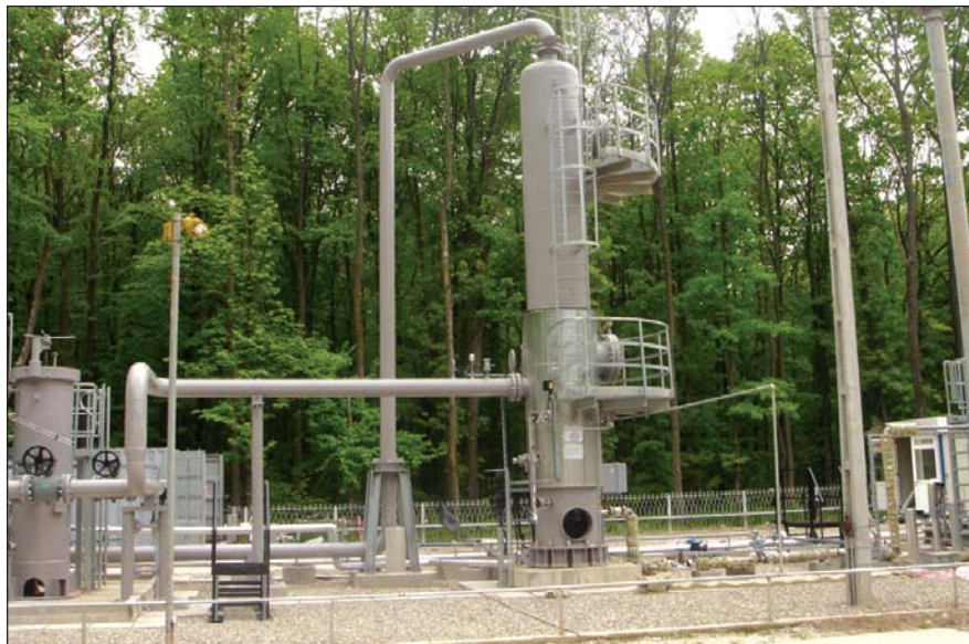
Accurate and reliable delivery of recovered glycol (TEG) to the top of the absorber vessel is critical at this final stage of gas drying.
