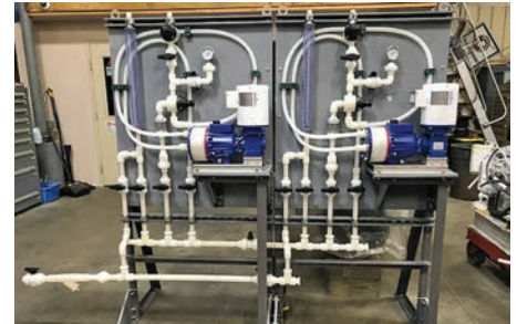
Dual P400 skid system with corrosion-resistant materials to meter Sulfuric Acid.
